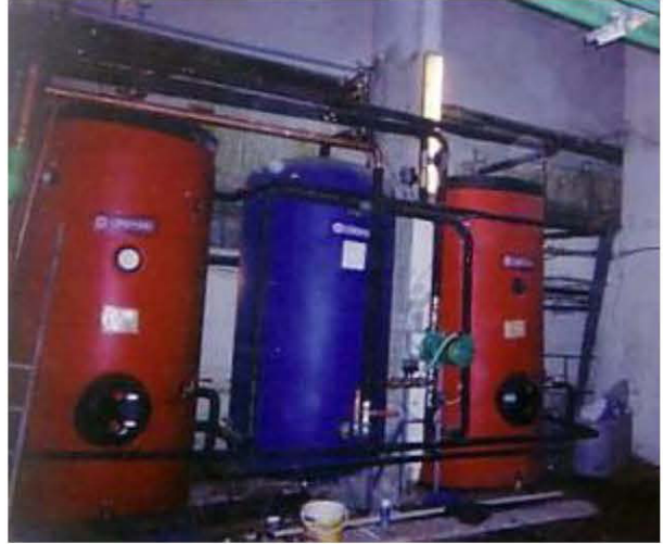
BOILER ROOM KONTOKALI BAY 3X3000 lit Boilers
