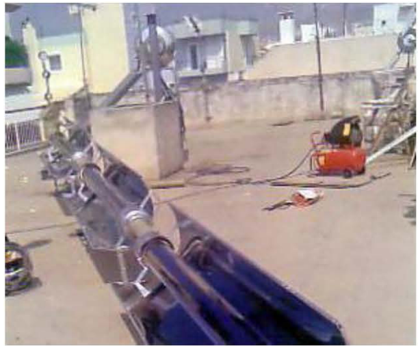
☆☆☆- CLOSED SIRCUIT MAG FOR STEAM PRODUCTION
